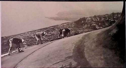
Work of cement finishers with their rhythmic trowels is a daring roof-brink ballet against uncertain background of merged sky and water; Elliott Bay shoreline far below.
