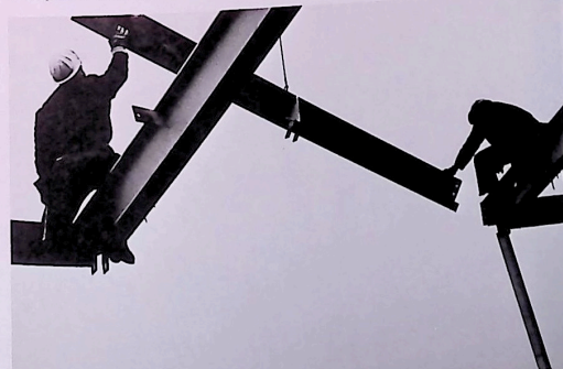
From their tip-end perch, ironworkers grapple for crane-sung piece to be placed along roof-brim.
