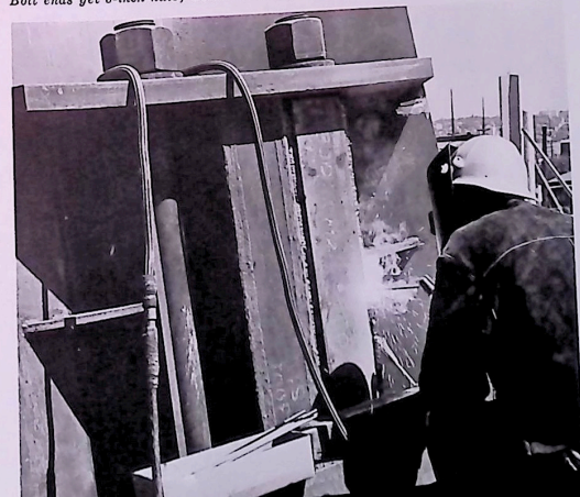
Bolt ends get 8-inch nuts; welders seal out the weather with solid steel.
