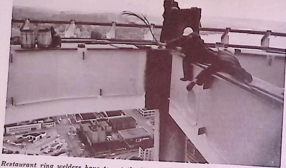
Restaurant ring welders have to get the line for their float down under that beam. I'll sling, you catch. Ground is 500 feet down.
