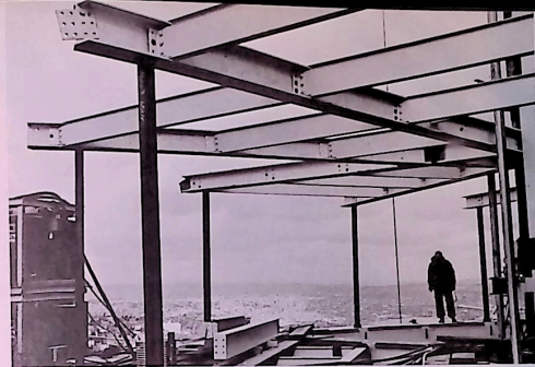
Robed for December blow, signalman Torrey on edge of restaurant deck contemplates last stages of an uncommon job. He has "talked" each Space Needle piece into place on his intercom to invisible crane operator below.
