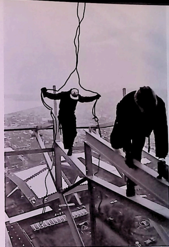
This 6-inch catwalk is limit of crane's reach; end pieces had to be slid out, with kneehold, by hand. Turtle-roofed Coliseum is no landing net below.
