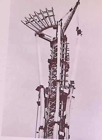
Thrill of restaurant perch takes on reality; third supporting arm is readied for next ring girder section.
