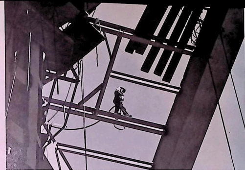
You walk where you have to go. Watch out for plank ends that are springboards to space.
