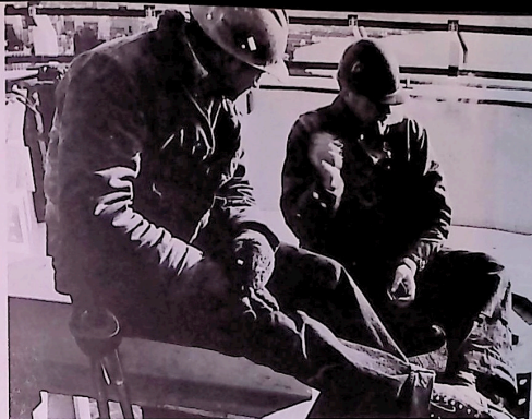
Waiting for new iron affords a moment of relaxation on restaurant beam.
