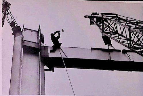
A meaningful blow of an "8-pound beater" on hole-aligning "drift pin" pegs the leg into place.
