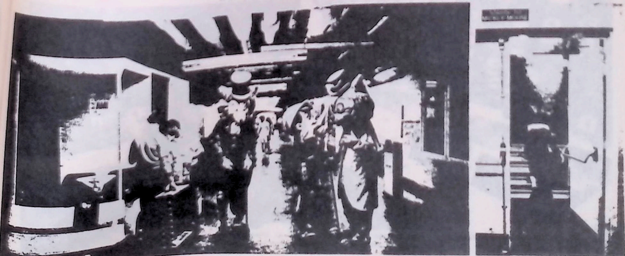
Down under: Between turns at strolling the grounds, costumed Disney characters (left) take a breather in the service basement that extends beneath the entire park; water, electric and sewage conduits run above their heads. Right, the star of the show heads upstairs to re-emerge in the Mickey Mouse Revue.
